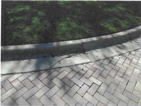
Minor concrete crack at curb and gutter
