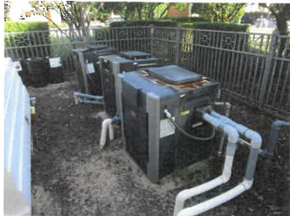
Rust at Carriage Point heater
