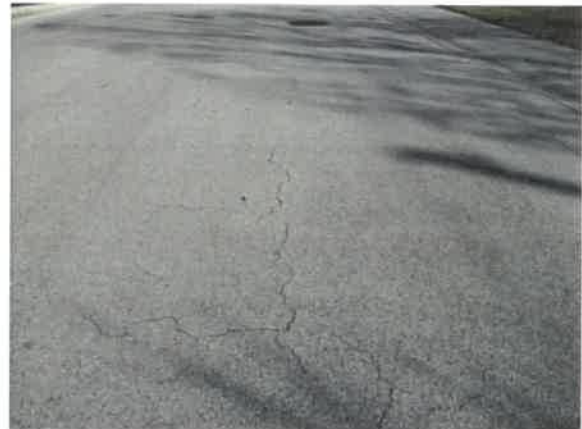
Minor cracks at Excitement Drive
