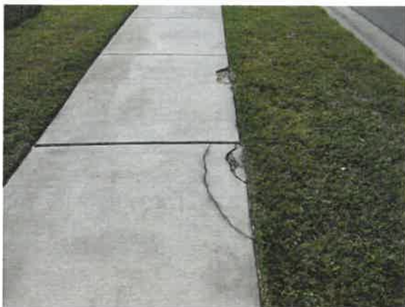
Concrete sidewalk cracks and damage
