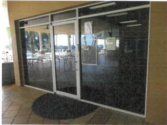
Aluminum frame window and door at Seven Eagles
