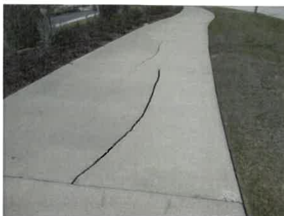
Sidewalk cracks near Tradition Boulevard gate house
