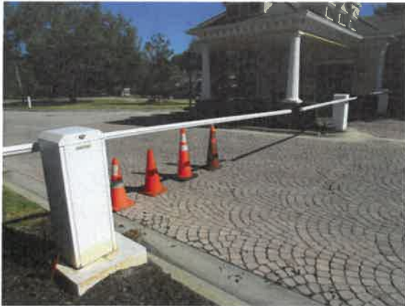
Gate arms and operators
