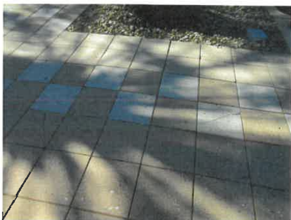
Isolated cracks at Seven Eagles
