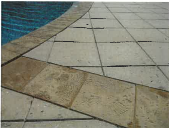
Minor paver lift at Heritage B
