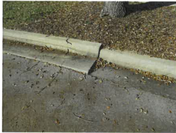
Settlement at curb and gutter
