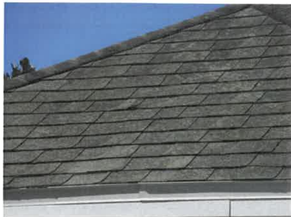
Shingle deterioration at Heritage B pool house
