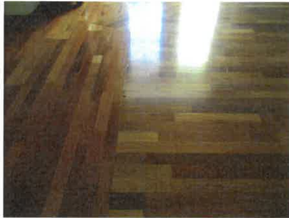
Minor deterioration at wood laminate floor
