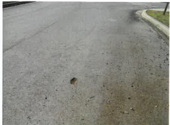
Example of minor damage
