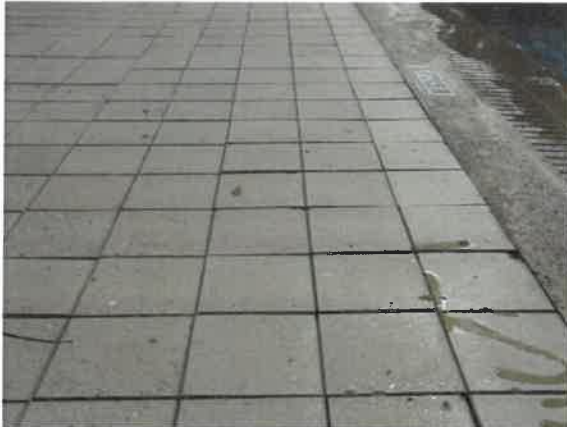
Spalls and minor settlement at Seven Eagles
