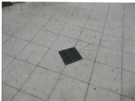
Cracked pavers at Carriage Point
