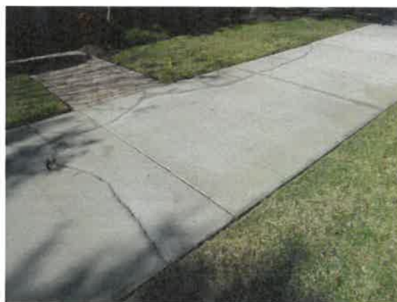
Multiple concrete sidewalk cracks near 1420 Reunion Boulevard
