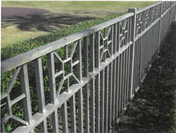
Typical aluminum fence, note fade
