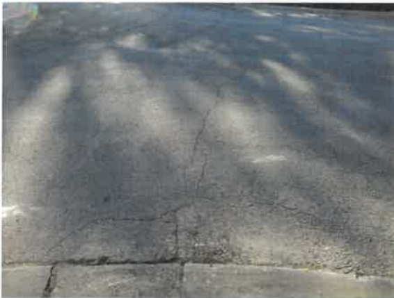
Minor cracks at Assembly Court
