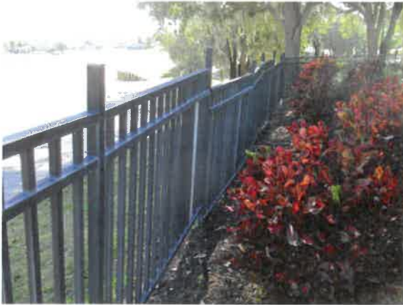
Leaning/loose section at Seven Eagles
