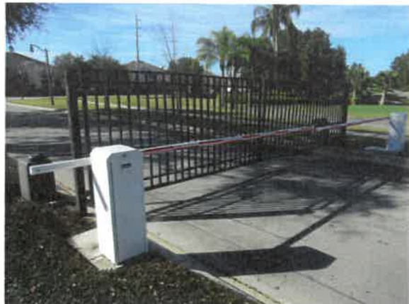
Gate arms and bi-parting gates
