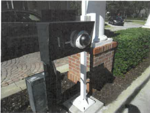
Main gate entry components
