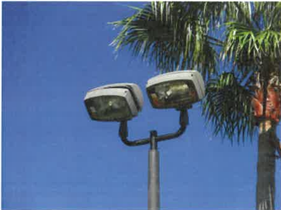
Loose fixture at Heritage B
