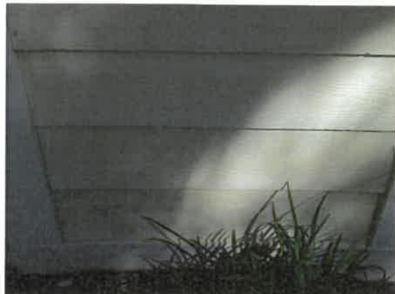
Finish deterioration at Heritage A pool house, note – budget for paint applications through operating budget
