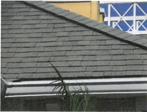
Granular loss at shingles at main gate house
